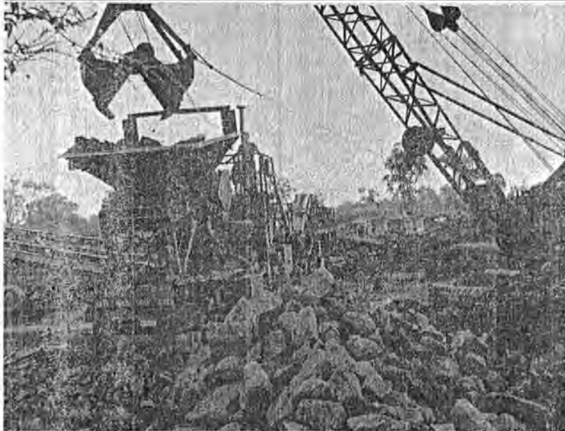
THE CRUSHER —A machine used for crushing rock into tiny stones is now in operation in the central highlands. It has helped to expedite the building of a road between Dak To and Ben Het by the 2nd Brigade. (USA Photo by PFC William Sigfried)
